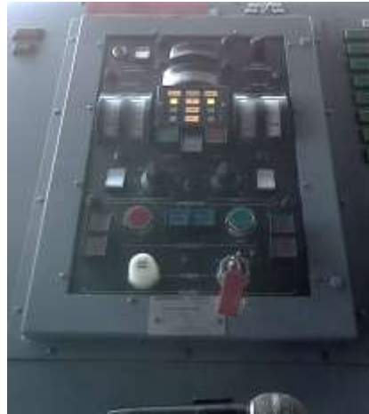
OLD ANALOGIC BRIDGE CONTROL PANEL
