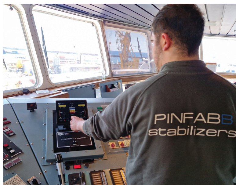
Pinfabb engineer onboard Mega Victoria during system testing
